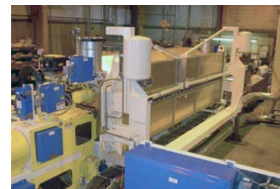
Blankwasher & Spray Lubrication System
